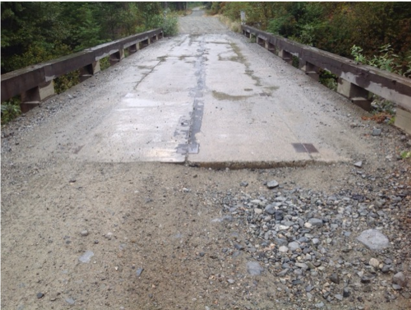
potholes at approach
