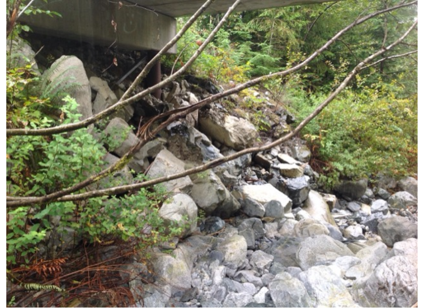
riprap scour on left bank
