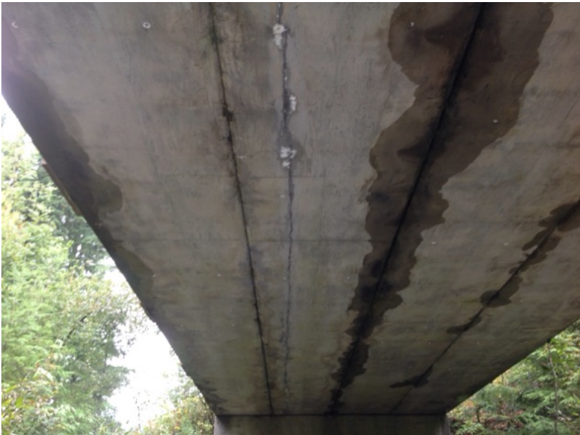
crack along underside of 3rd slab - no apparent change
